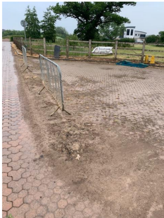
Surface mud on thrid exit of roundabout
